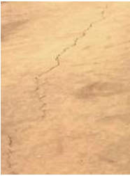
Illus. 2: Crack in a ceramic surface
