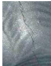
Illus. 5: Fracture in a welded joint
